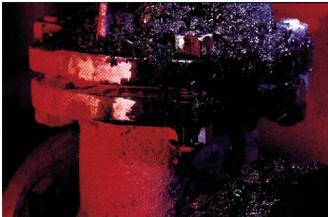
Use of heat transfer fluid with a high vapour pressure can lead to heavy sludge build-up around control valves and pipe flanges.
